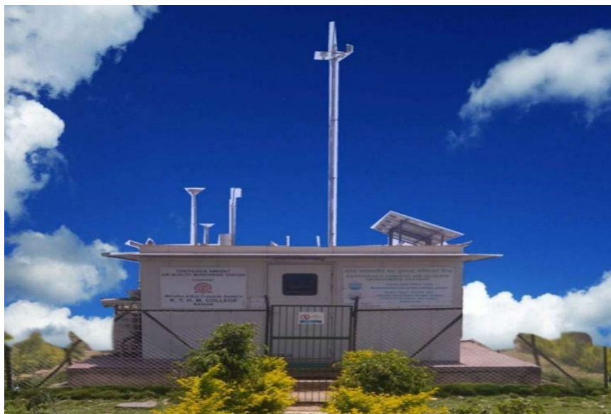
Continuous Ambient Air Quality Monitoring Station (CAAQMS)
