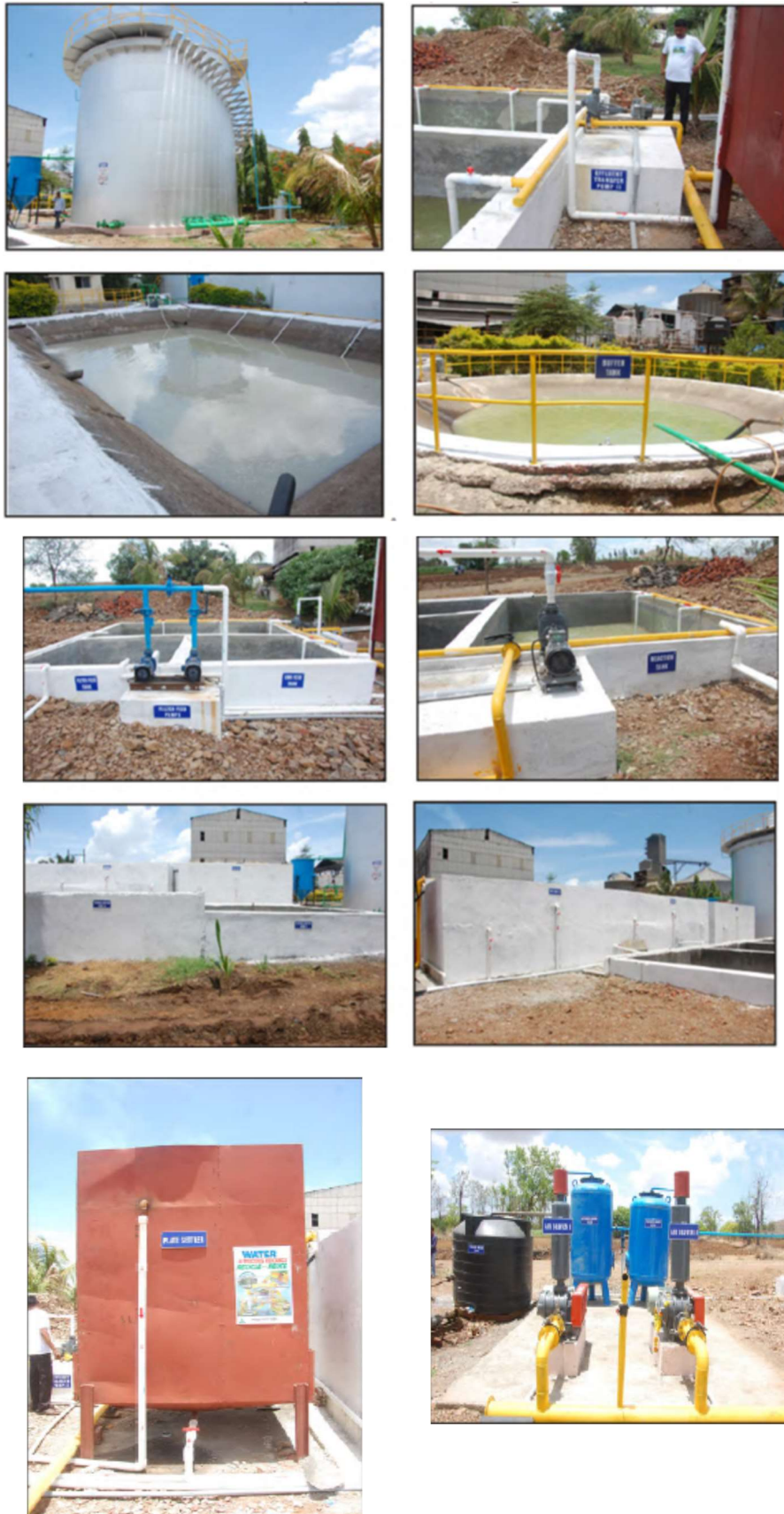
Figure 3 Existing Upgraded ETP On Site
