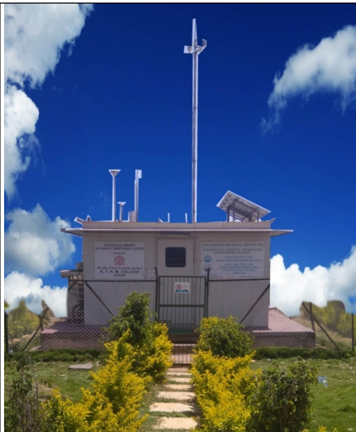
Continuous Ambient Air Quality Monitoring Station
