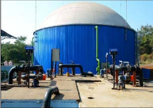
Advanced Waste Management Plant
