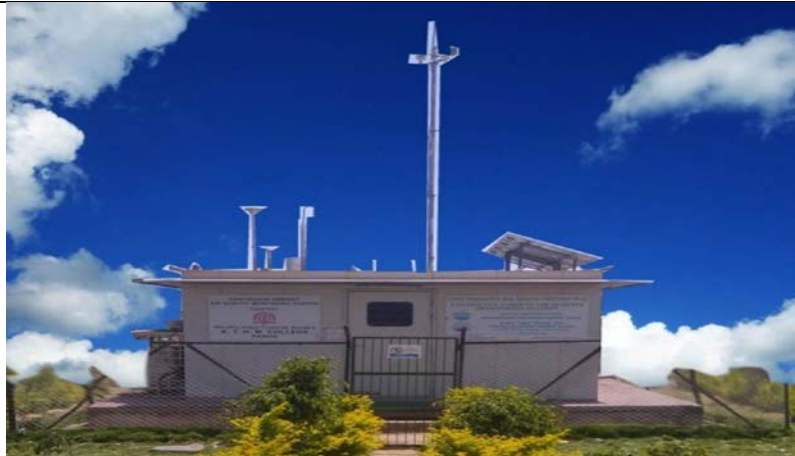
Continuous Ambient Air Quality Monitoring Station (CAAQMS)
