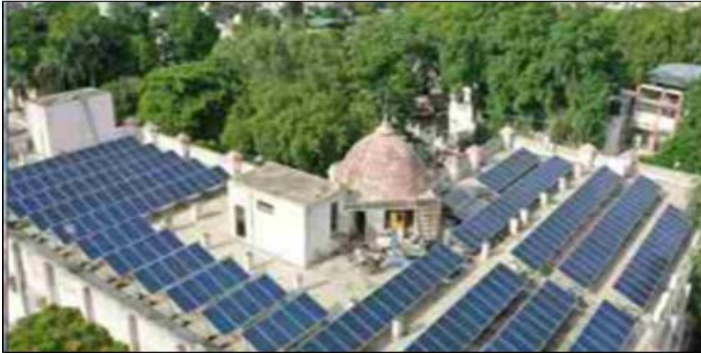
Solar Roof Top
