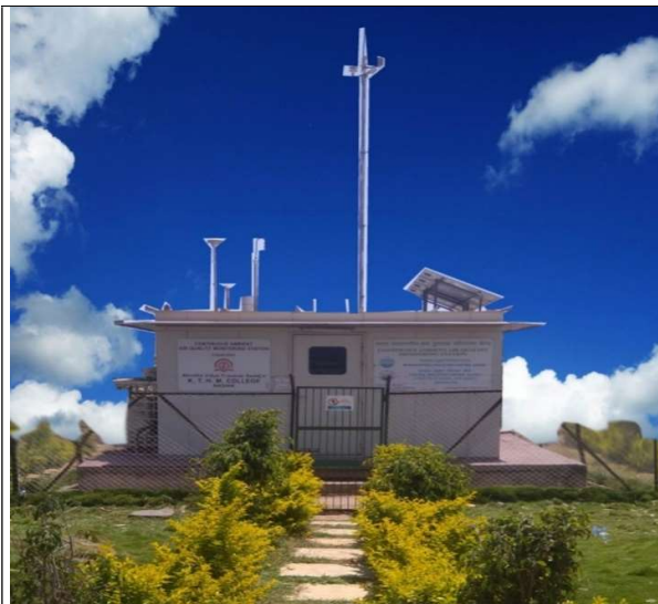
Continuous Ambient Air Quality Monitoring Station (CAAQMS)
