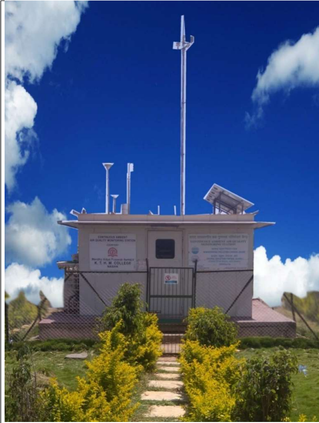
Continuous Ambient Air Quality Monitoring Station (CAAQMS)
