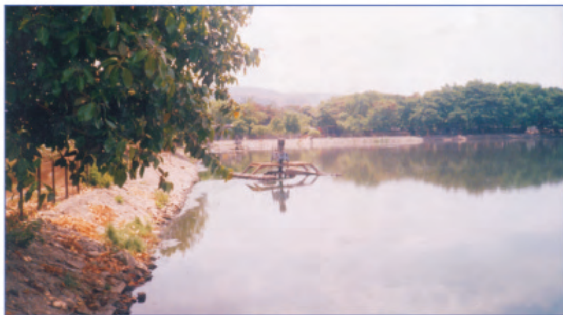
Fig. 6. Non-functioning aerator at Airoli Sewage Treatment Plant
